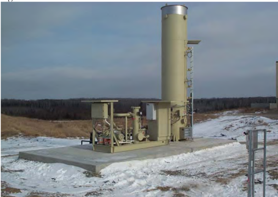
Figure #2: Enclosed Flare
